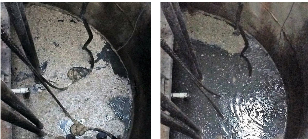
Figure 2. A municipal lift station with fats, oils, and grease (FOG) coverage over most of the surface of the water (left) was treated with Biotifx®. After treatment most of the surface of the water was cleared of FOG (right).
